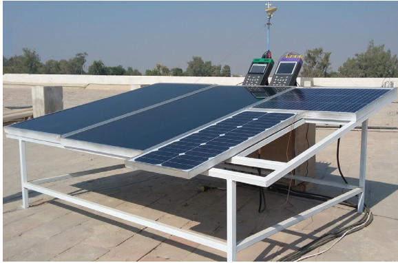
Figure 1. Experimental setup including modules, data loggers and weather station
