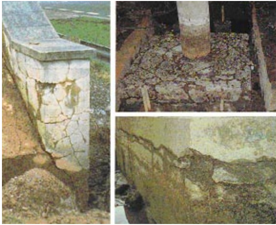
Fig.1. ASR Pattern Cracks [23].
