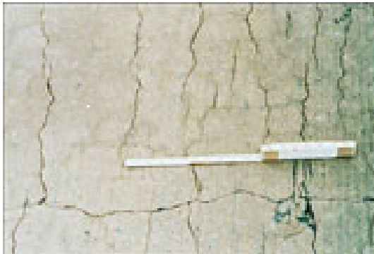
Fig.2. ASR Pattern Cracks with a Longitudinal Trend in a Concrete Pavement [23].
